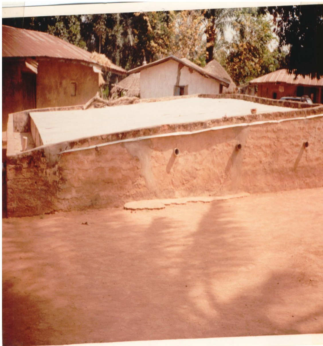
Plate VI: A Community Rainwater Harvester Tank in Obijiago Community, Obi LGA.
