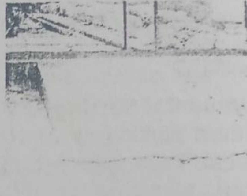
Figure 6. Ramp without Handrails
