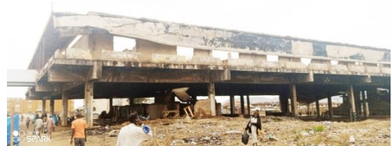
Figure 5: Jos Main Market Terminus, the current state. (The Relic and the Ruin)
